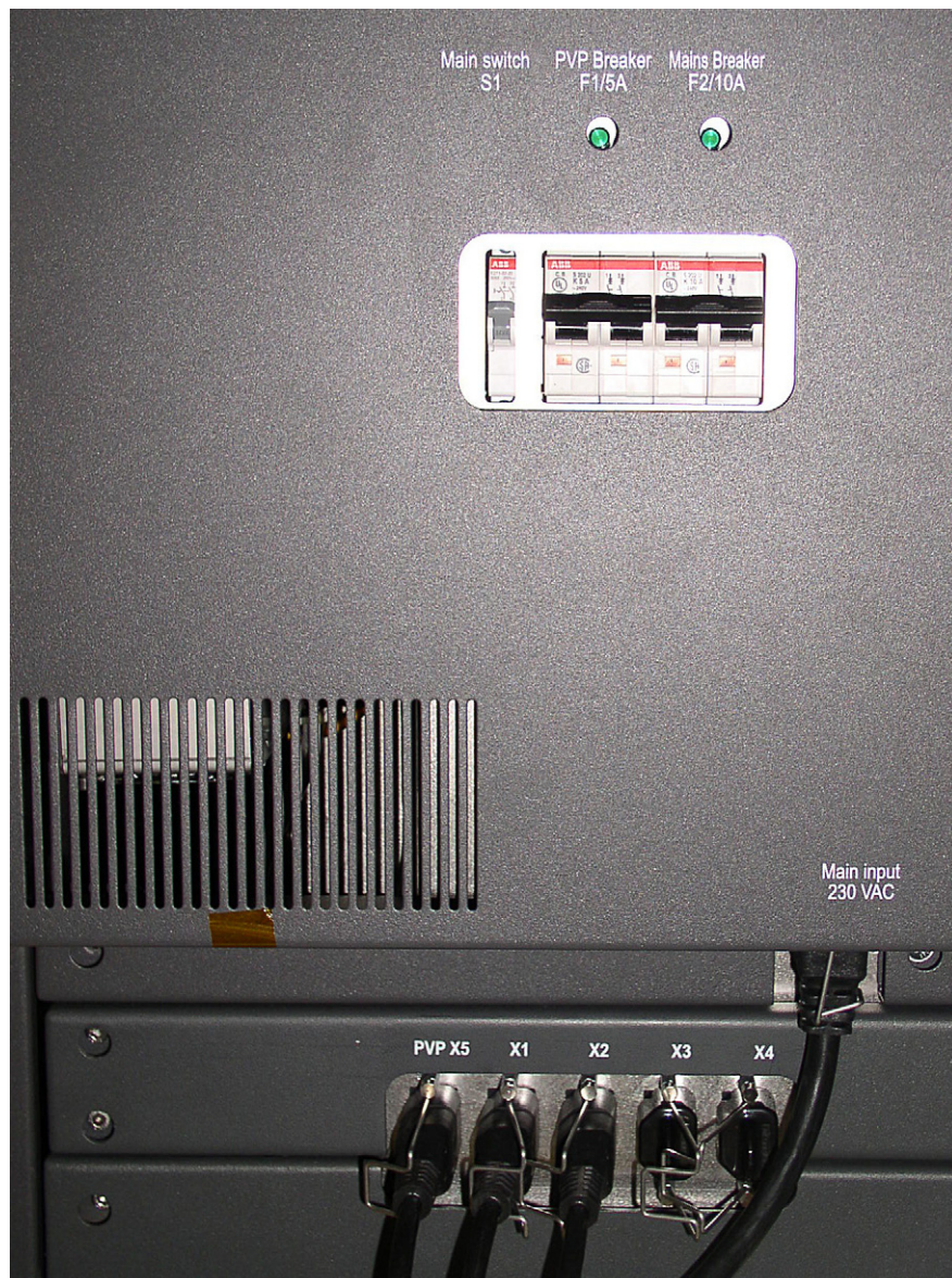
FIGURE 2-3: Mains switch board
